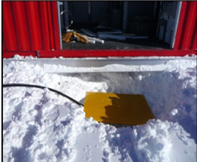
Figure 14.7 Grate covering hole
