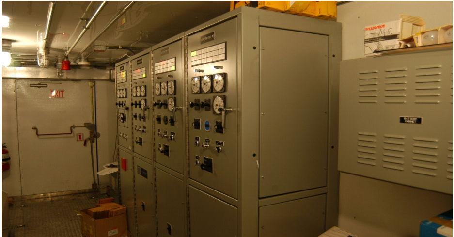
Figure 2.9 Power Distribution Module (PDM) interior
