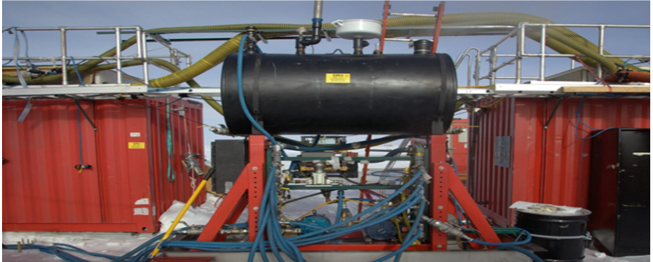
Figure 2.95 Fuel tower/ day tank
