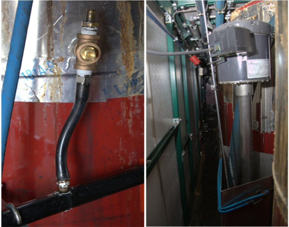
Figure 2.124 Condensate drain cross fitting and drain tubing on model 75 (left) and condensate tank with submersible pump (right). The blue hose entering the condensate tank comes from the Y-strainer manifold.
