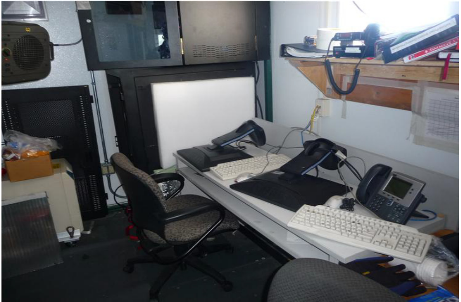
Figure 12.13 Improperly secured drill control room
