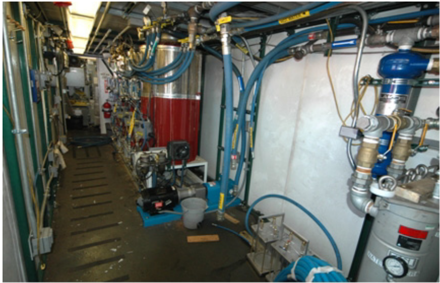
Figure 2.37 PHS interior view
