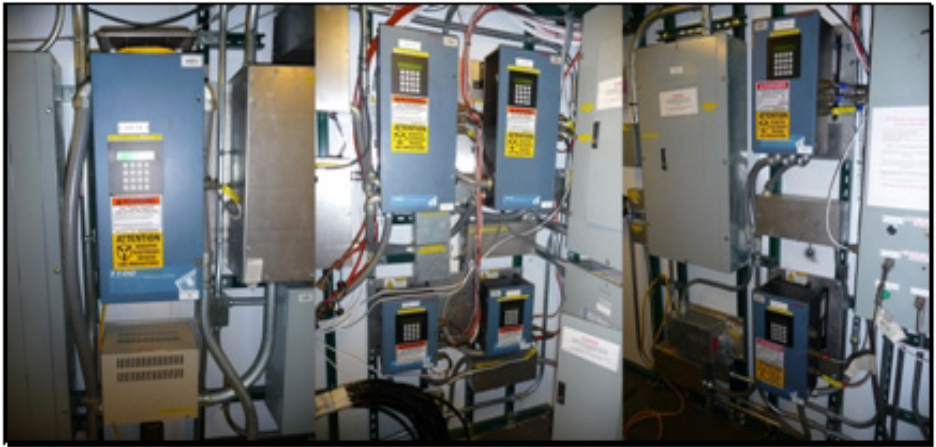
Figure 12.3 Motor drives in TOS electrical closet
