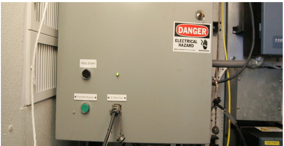
Figure 5.9 E-Stop enclosure where the E-stop cable enters from the side of the closure
