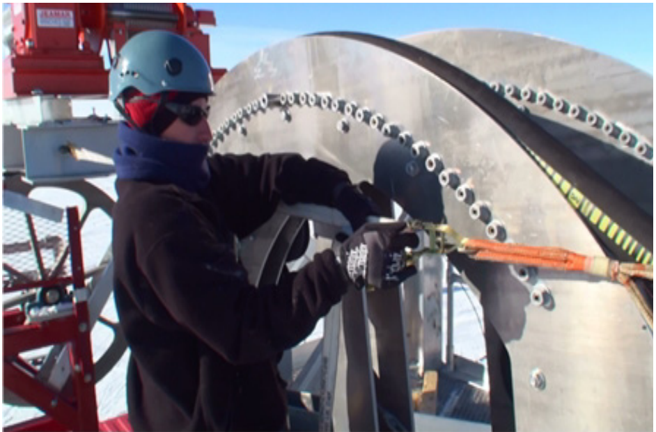
Figure 9.8 Anchoring the main hose on the tower via the attached Yale Grip
