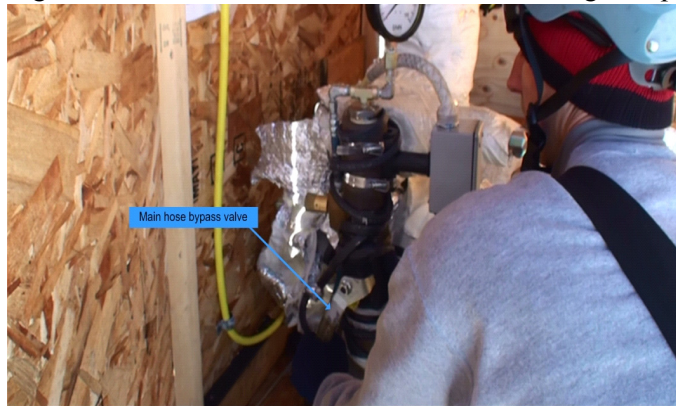
Figure 9.34 Main hose bypass valve being opened to connect main hose to drill head
