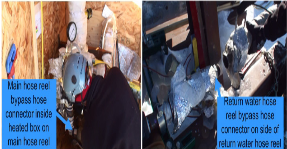
Figure 9.5 Bypass hose being connected to main and return water hose bypass valves
