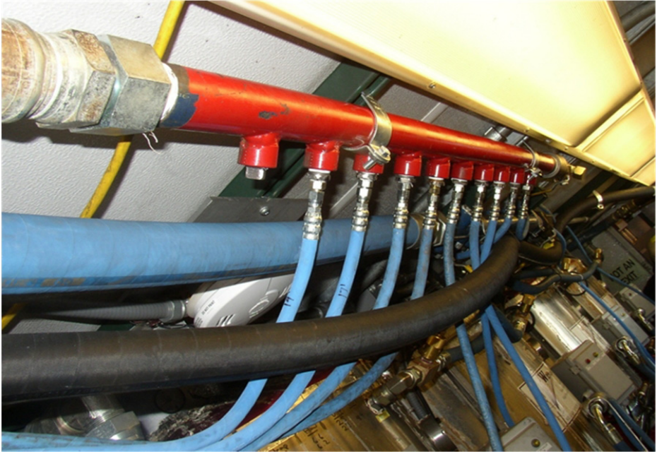
Figure 2.125 Y-strainer centralised manifold on ceiling of MHP building
