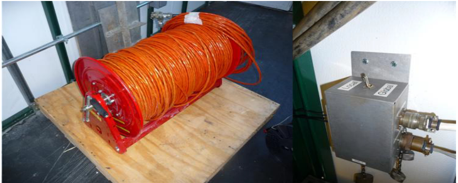
Figure 12.16 Network cable and TOS network junction box
