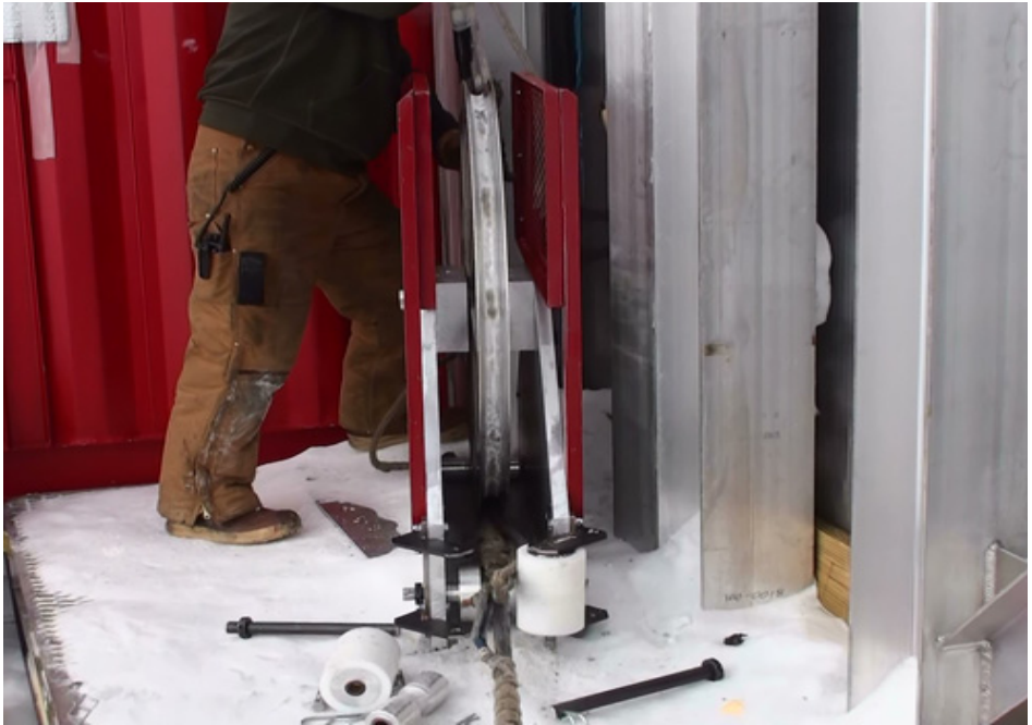
Figure 9.11 Tower floor cable sheave showing guide rollers
