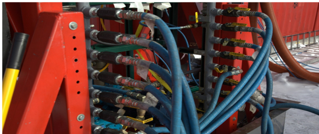
Figure 2.96 Fuel tower feed manifolds
