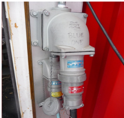
Figure 14.24 Tower hoist power connectors
