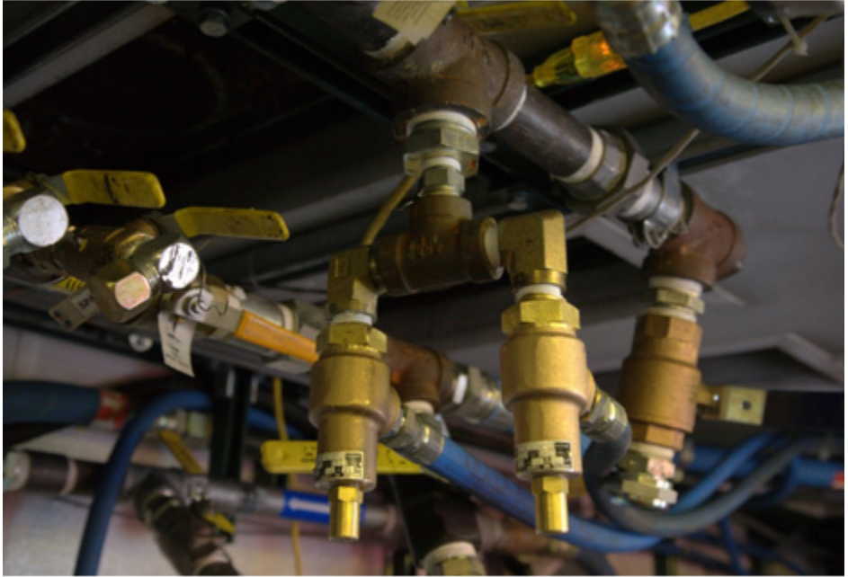
Figure 6.10 PHS Heater PVR's
