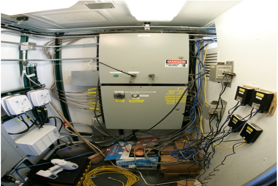
Figure 5.10 DCC utility closet showing the breakout boxes to the right.
