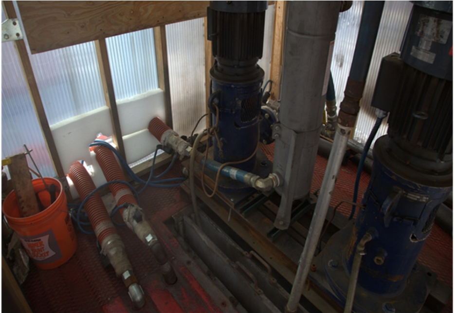
Figure 15.7 Vertical turbine pumps and filter
