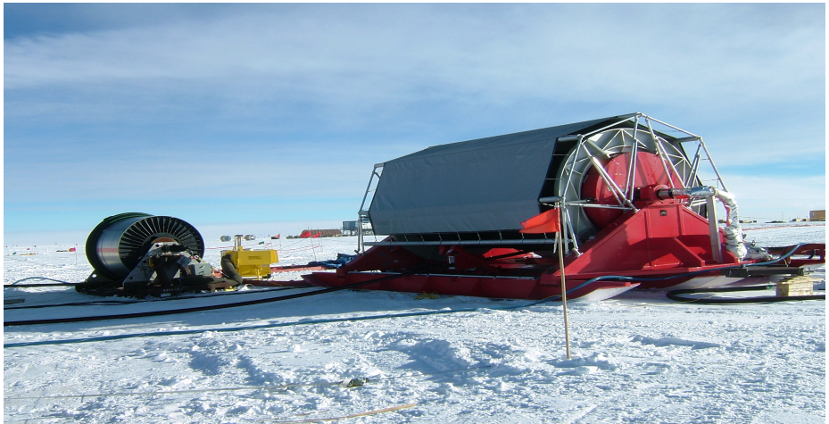
Figure 2.103 Main supply hose reel to the right. Return water hose reel is to the left
