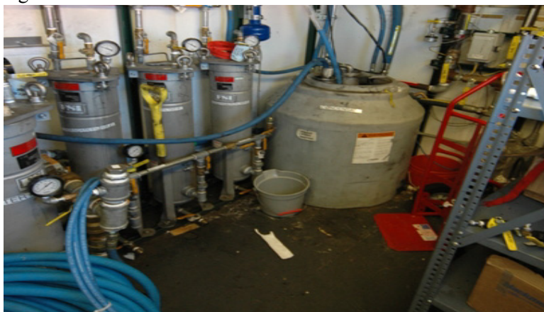
Figure 2.39 Condensate collection and filtration system inside PHS.
