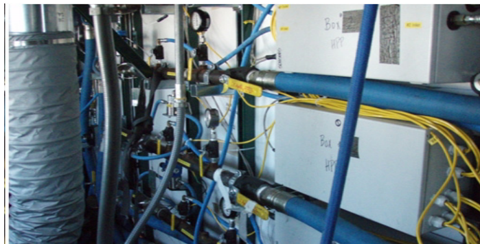
Figure 15.11 HPP pump manifold
