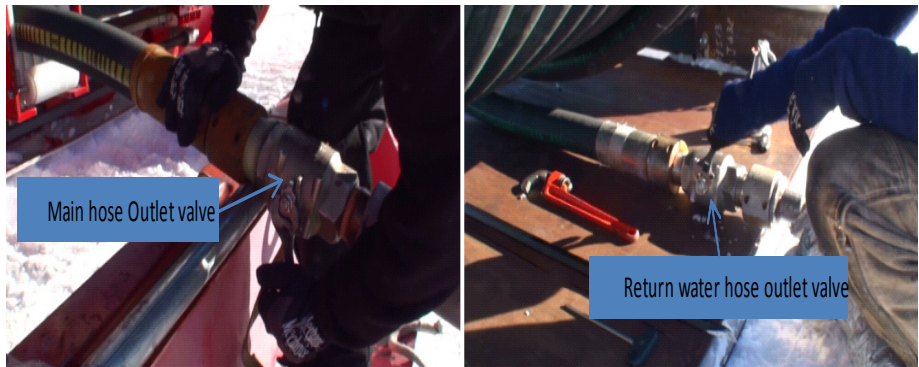
Figure 9.3 Main and return hose outlet valves being closed for routing into tower
