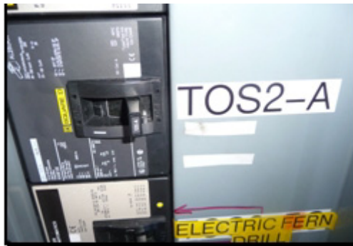
Figure 14.4 TOS circuit breaker at PDM
