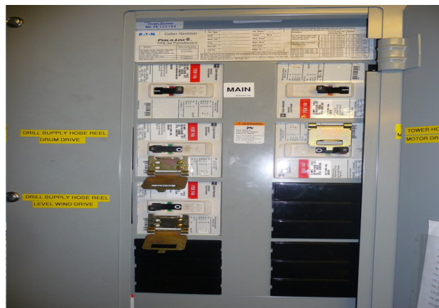
Figure 14.3 TOS main circuit breakers at the top of the breaker panel
