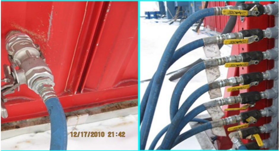
Figure 5.1 Photos showing fuel connection point on MHP and fuel tower
