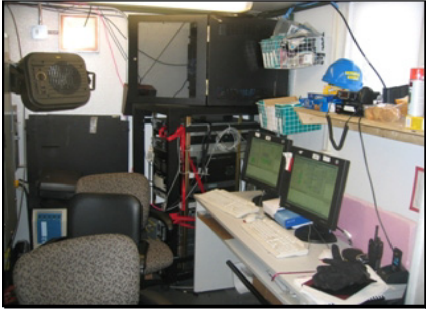
Figure 14.19 TOS drill control room in operational state
