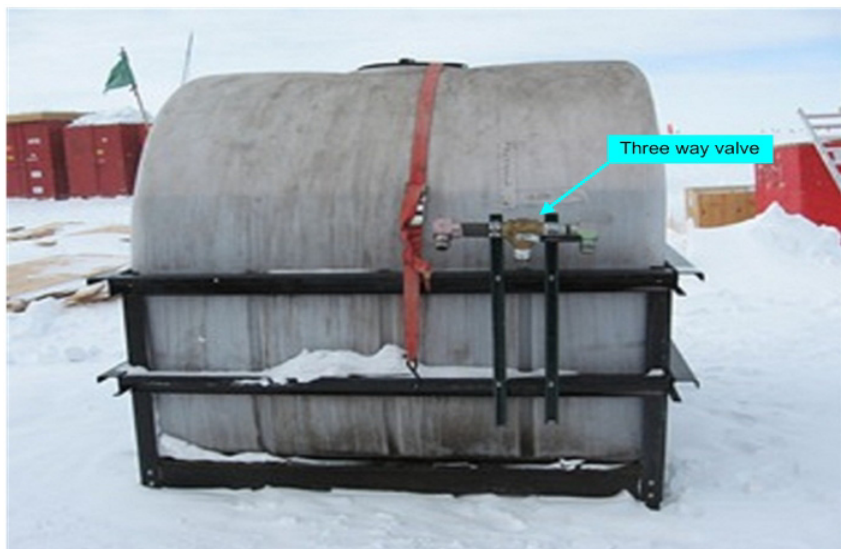
Figure 15.4 800 gallon glycol tank with 3 way valve
