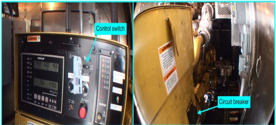
Figure 15.16 Generator control switch and circuit breaker locations
