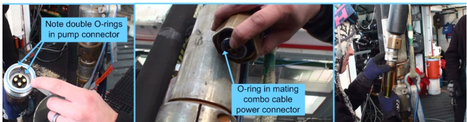
Figure 9.57 Inspecting pump power and combo cable mating connectors for O-Rings
