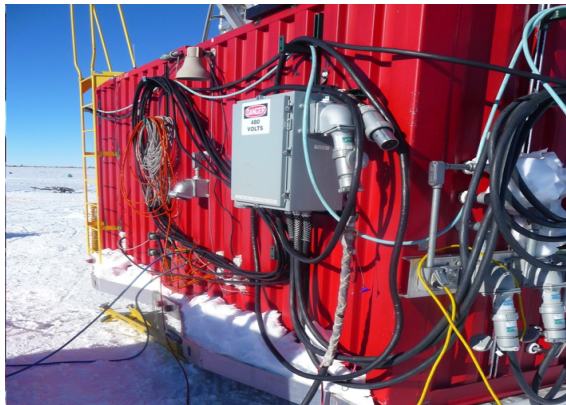
Figure 14.5 TOS power interface box
