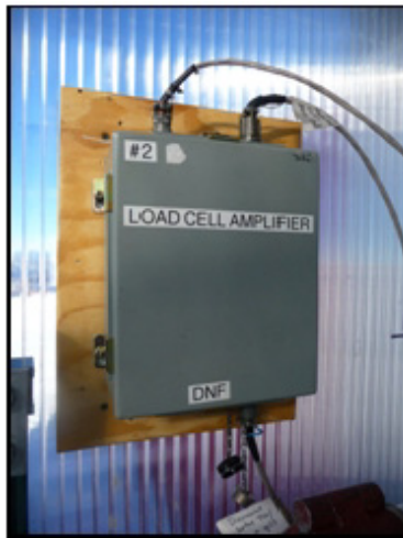
Figure 12.15 Load cell amplifier box with cable to be disconnected at bottom of box
