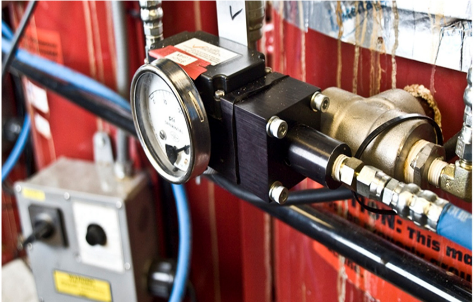
Figure 2.121 Differential pressure gauge and switch
