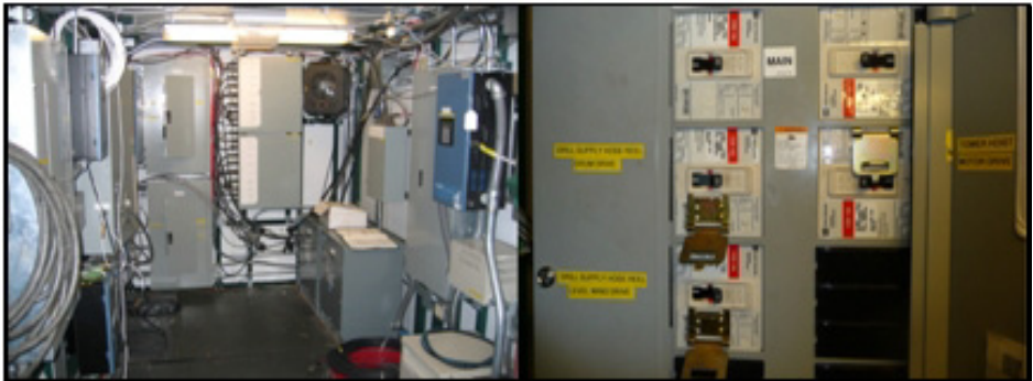
Figure 12.2 TOS electrical closet and main circuit breaker
