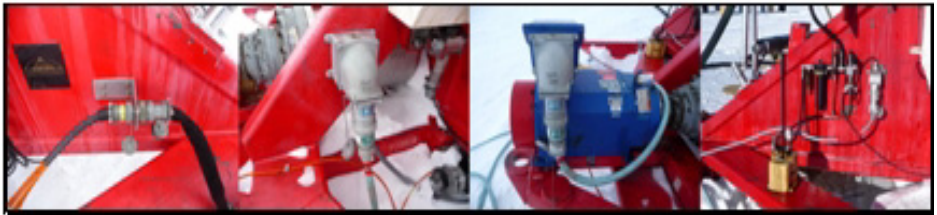
Figure 12.4 DSHR cable connectors (network, level wind, drum and brake cables)
