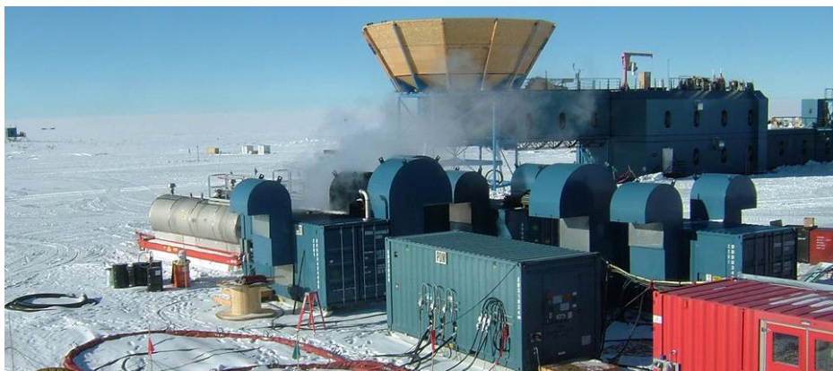
Figure 2.22 View of the 3 generators, with the PDM in the foreground
