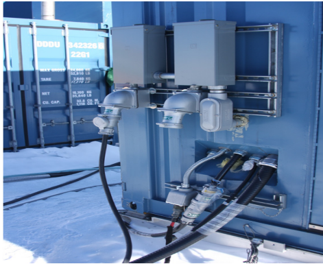
Figure 15.18 Generator feed cable
