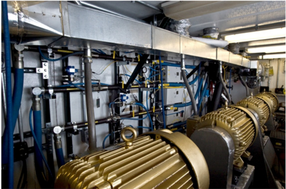
Figure 2.57 Inside HPP building showing pump motors and plumbing wall
