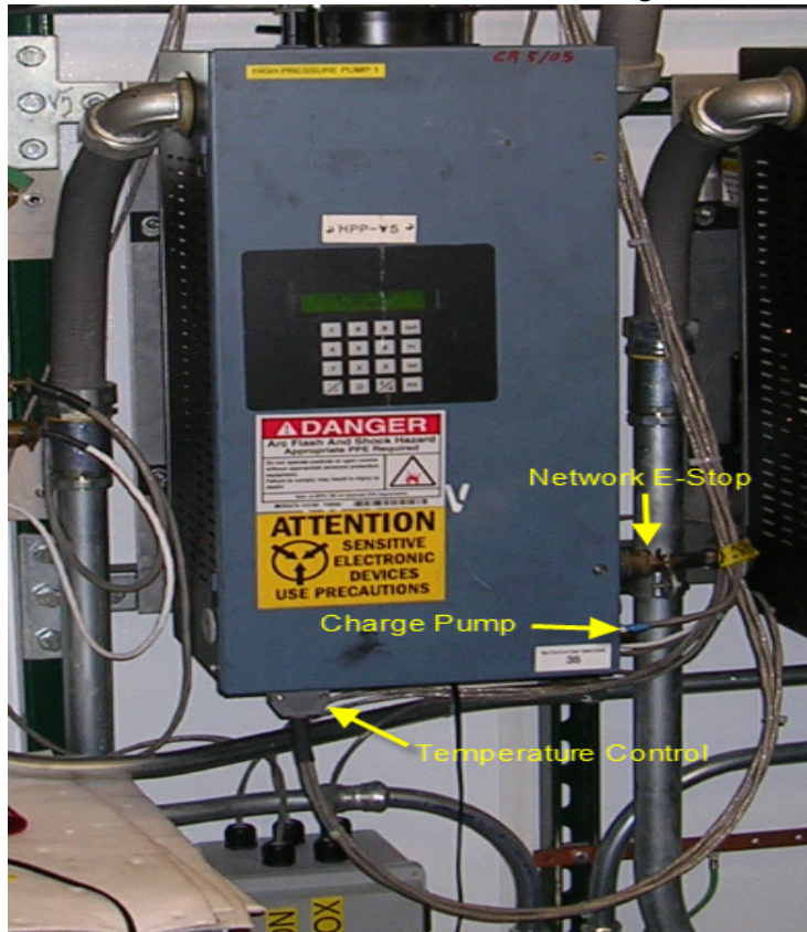
Figure 3.3 HPP motor drive showing the Network, charge pump and temp control connections
