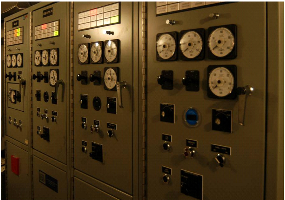
Figure 2.25 PDM switchgear cabinets
