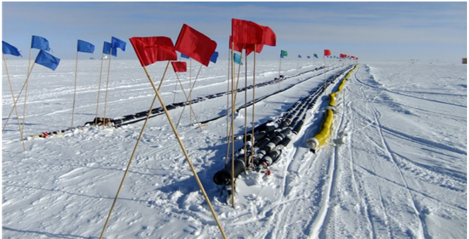
Figure 15.6 Surface and jumper hoses laid out and flagged for winter storage
