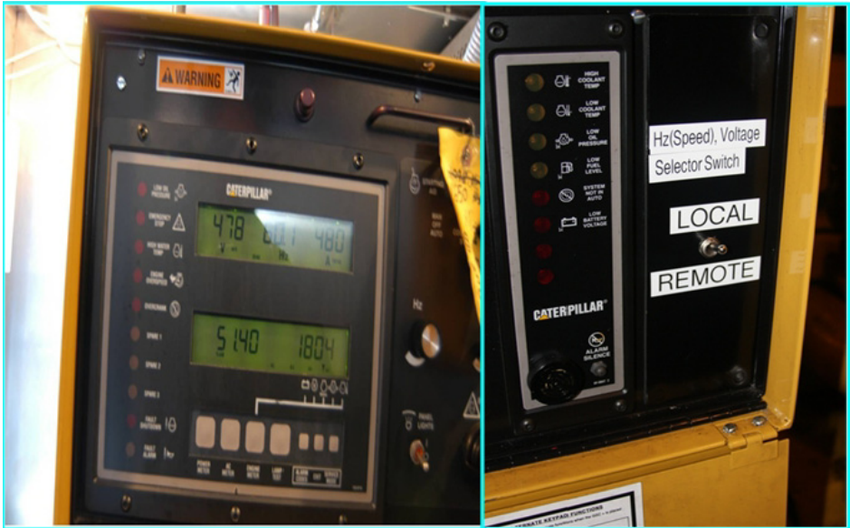
Figure 2.24 Caterpillar generator EMP-II control and “LOCAL/ REMOTE” switch
