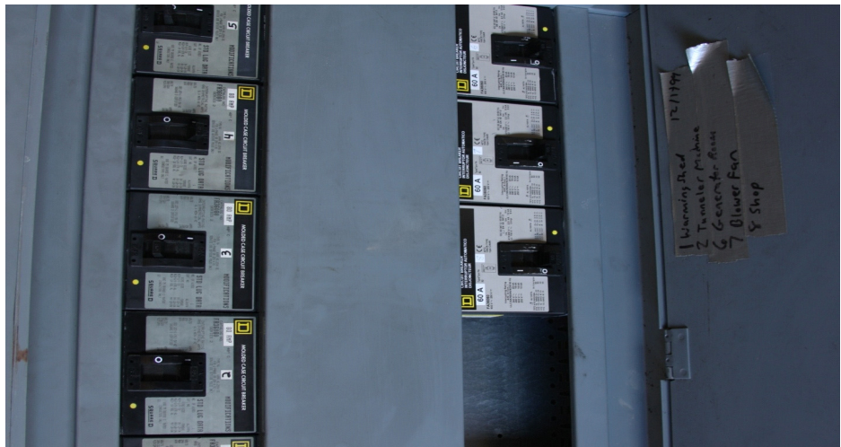
Figure 2.10 Individual MDS circuit breaker panels inside PDM
