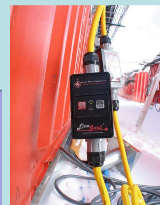
Close-up of GFCI module
