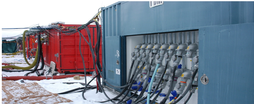
Figure 2.12 PDM power distribution panel showing feeder cables leaving to MDS'
