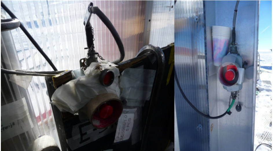
Figure 14.14 E-stop cables connected to tower inside and outside slap buttons
