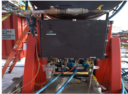
Figure 2.97 Control box at end of fuel tower
