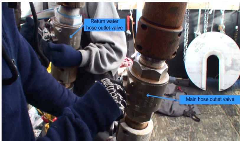
Figure 9.35 Closing main and return hose outlet valves to disconnect the coupler
