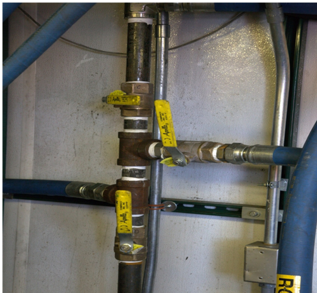
Figure 15.15 Booster pump bypass valve
