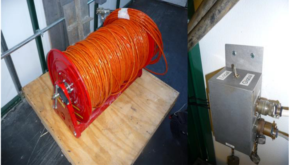
Figure 14.16 Network cable attached to network box inside TOS electrical closet
