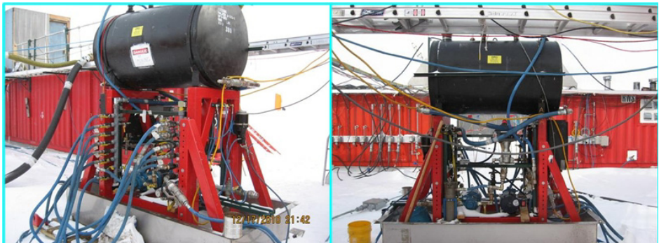
Figure 5.2 Fully plumbed fuel day tank
