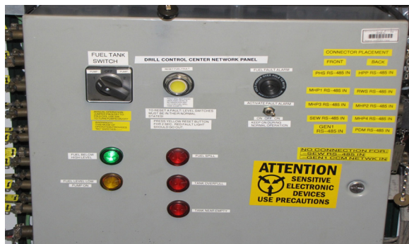
Figure 2.98 Fuel tank controls mounted on network panel inside DCC
